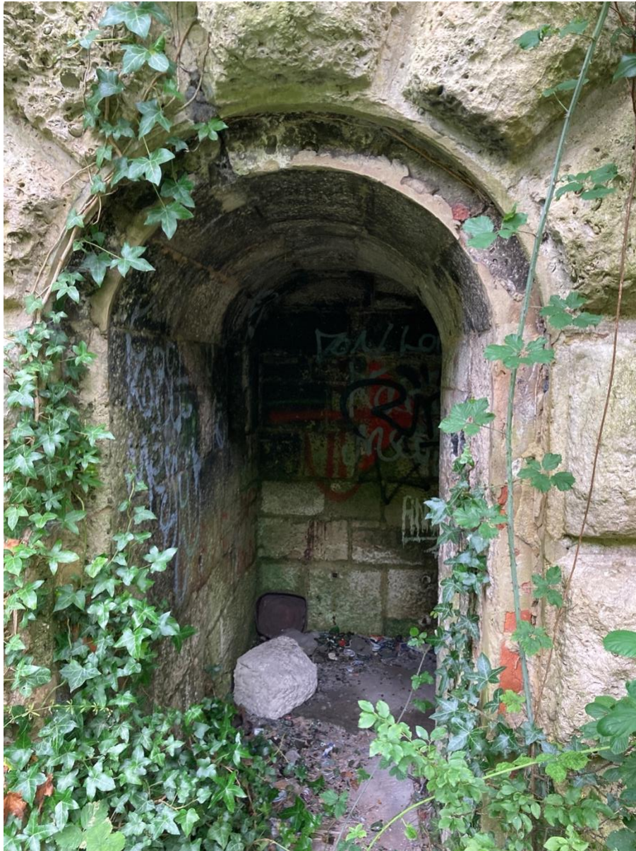
Figure 8: A photo showing the entrance to a tunnel. Brambles and ivy grow up and over the stone walls. A block of white stone sits at a slight angle away from the wall just inside the entrance to the tunnel. Graffiti covers sections of the inner walls.
